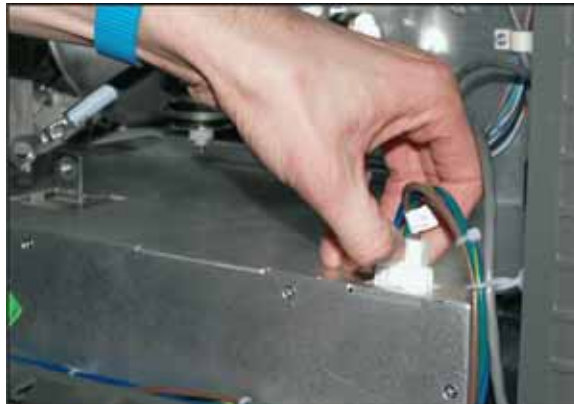
Figure 5-27 AC Power Harness
